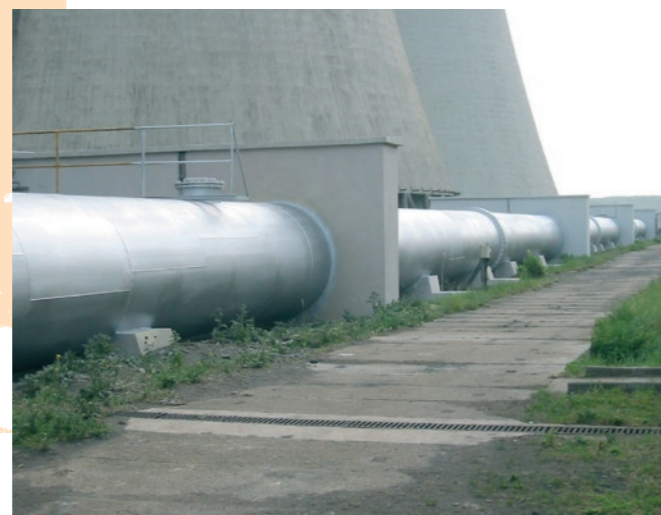
Potrubi po aplikaci antikorozičního systému Piping after the application of the anti-corrosive system
